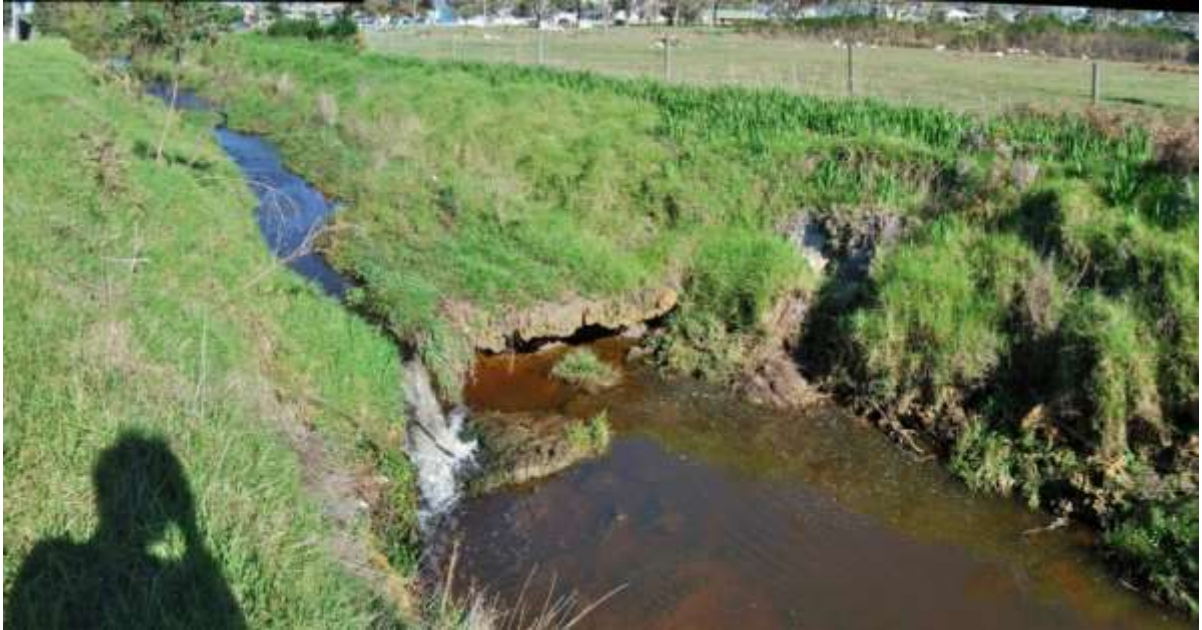
Figure 3: The waterfall and head-cut a short distance downstream of the North Road and Sanford Road intersection. The upstream progress of the head-cut has been slowed by a coffee rock layer.
