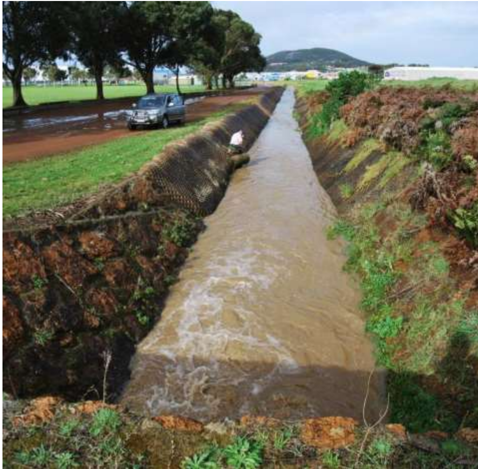
Figure 12: The armoured section of Yakamia Creek at the western end of Centennial Park Sporting Precinct, July 2011.
